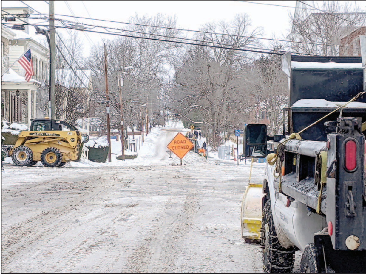
Public works crews closed several roads through downtown on Monday morning in order to finish their overnight project of clearing snow. (Photo by Adam Pack)
