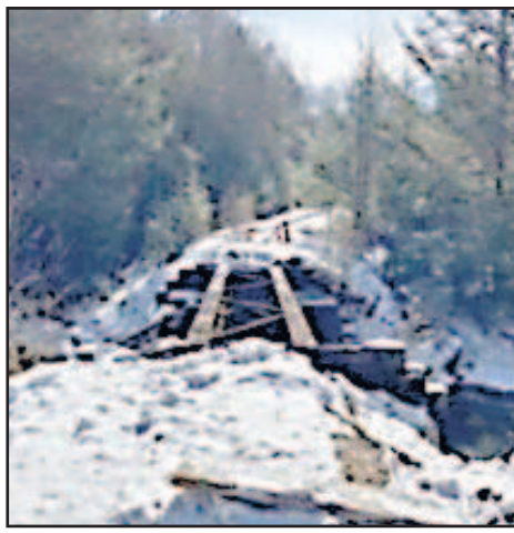
Damage on the Russellville Bridge
