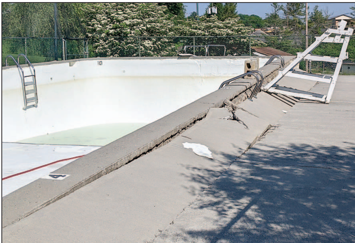
Pool lifted out of its frame, deep end first, cracking the concrete and causing major damage
