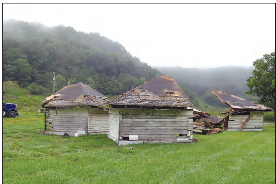
The roof is pictured here lying adjacent to the pavilion (Cathy Bolt photo)
