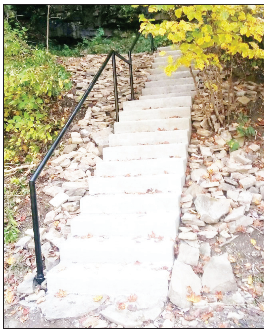
These new river access steps near Anthony provide a safer way for visitors to traverse a slope down to the Greenbrier River.
