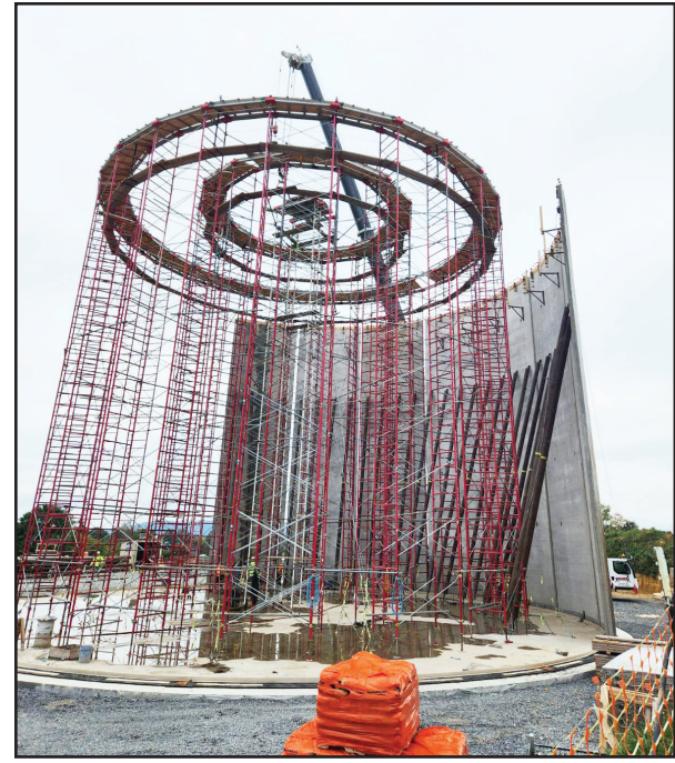
The new Yates water tank progress is shared here in a photo released by the City of Lewisburg.
