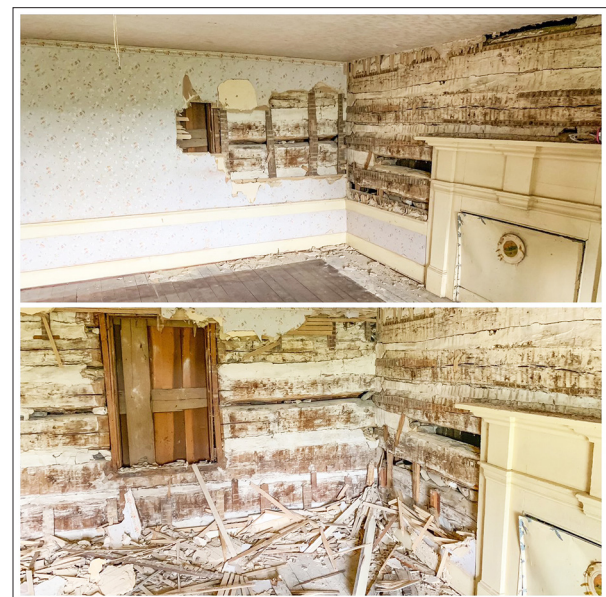
The extensive plaster removal process was arduous, but revealed a stunning history of the home and fort.
