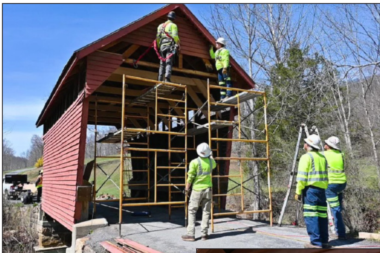
The historic Laurel Creek covered bridge was repaired earlier this week after apparently being struck by an oversized truck.
