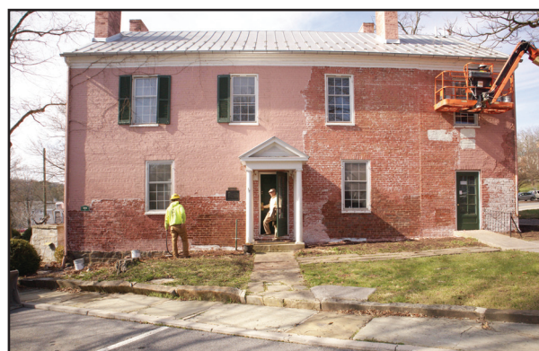
Al Emch, President of the Greenbrier Historical Society, stands in the doorway of the 1834 Supreme Court of Appeals of Virginia Law Library while conferring with a worker from Buckeye Construction.
