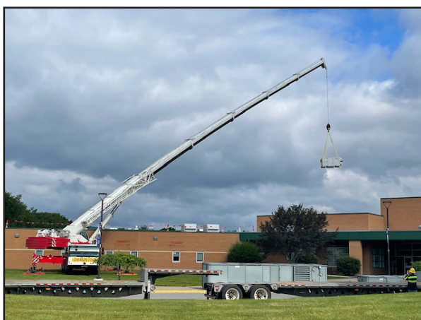
A new HVAC unit is lowered onto the roof of Western Greenbrier Middle School as part of an energy savings program adopted by Greenbrier County Schools. (Photo by RealWV)
