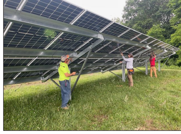
Workers string together solar panels behind Rupert Elementary School. (Photo by RealWV)
