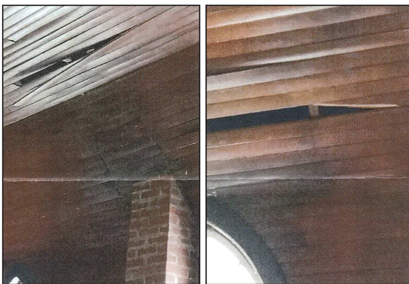
Interior of Ketron Church in need of repair
