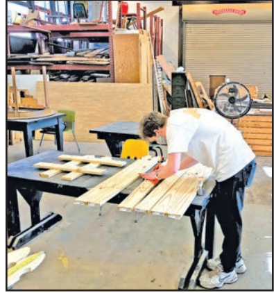
Building trades student Ryan Gordon measures out the components for the Glencoe Mansion snowflakes before cutting.
