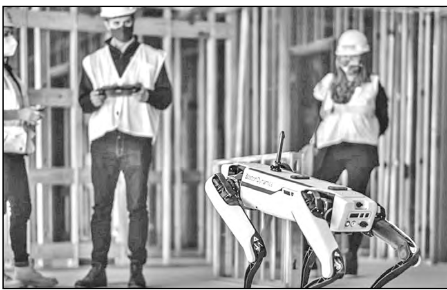
Virginia Tech researchers, students, and industry leaders, pictured inside the Creativity and Innovation District residence hall job site, are testing out Spot, a robotic dog, to monitor construction progress on the Virginia Tech Blacksburg campus. Photo by Sarah Myers for Virginia Tech.
