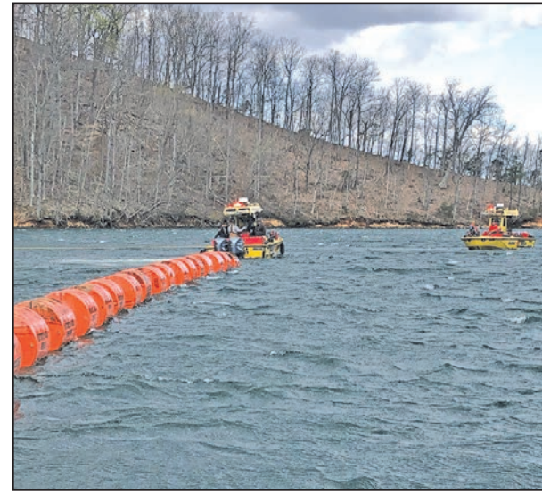
High winds and waves Friday night broke the floating boat barrier that keeps boaters away from the intake side of Smith Mountain Dam.
