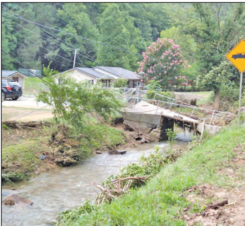
Severe flood damage near Isom, Kentucky. Photo courtesy of Elaine Tanner of Friends for Environmental Justice.
