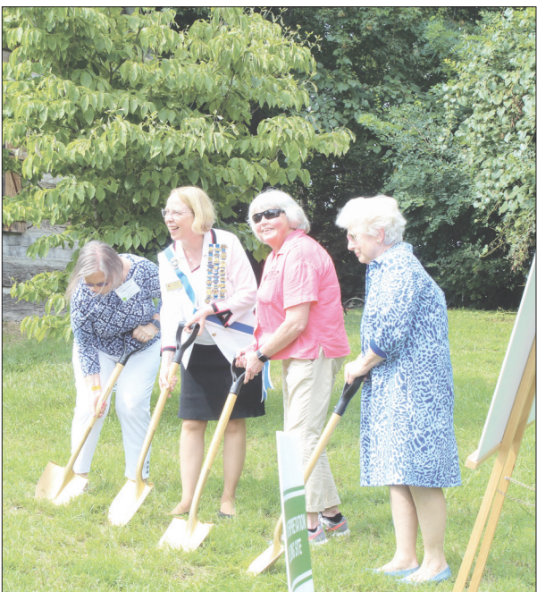
Peggy Fanney, LeAnn Turbyfill, Laura Wedin and Joann Sutphin break ground with golden shovels.
