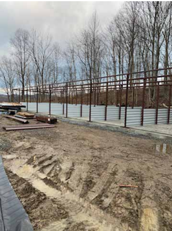
A second location for Eagle Storage (in Shinnston) is underway but with work still to be done. Weather permitting, they are hoping construction will be complete this month with rentals available by January 1st.
