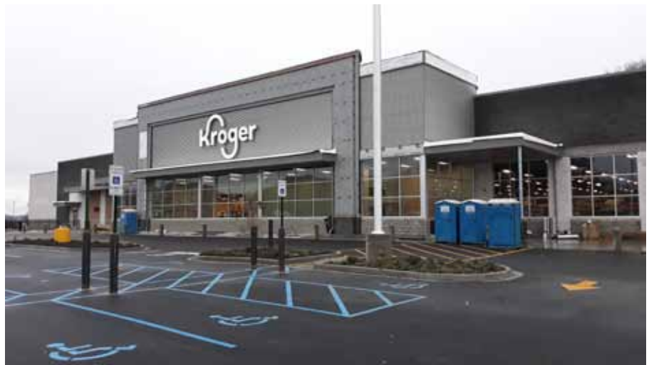
Crews are working round the clock on the interior of the new Kroger facility at Eastpointe in Clarksburg. The new, expanded store is 50% larger than the existing Kroger and will offer more to customers including drive-thru pharmacy pickup. The larger space will also necessitate an increase of up to 50 more employees.
