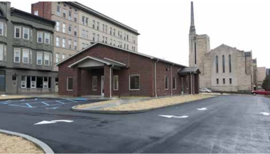
Work progresses at the new Post Office location in downtown Clarksburg. Striping has been completed in the parking lot and driveway markings show that traffic can exit or enter from either Pike or Main Streets.
