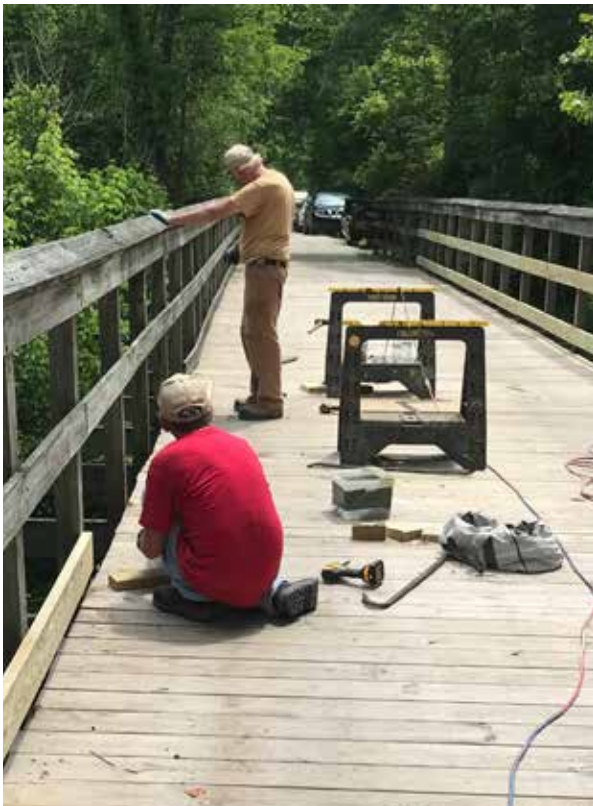
Pictured here, NBRTF volunteers work on replacing weathered decking and railings along some of the Rails to Trails bridges. Funding is requested to continue this work.
