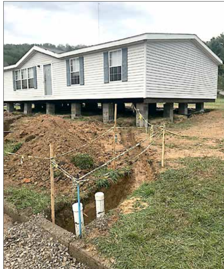
The Progressive Women's Association helped find a family in need of shelter and provided them with this home, which first needed the construction of a secure foundation.
