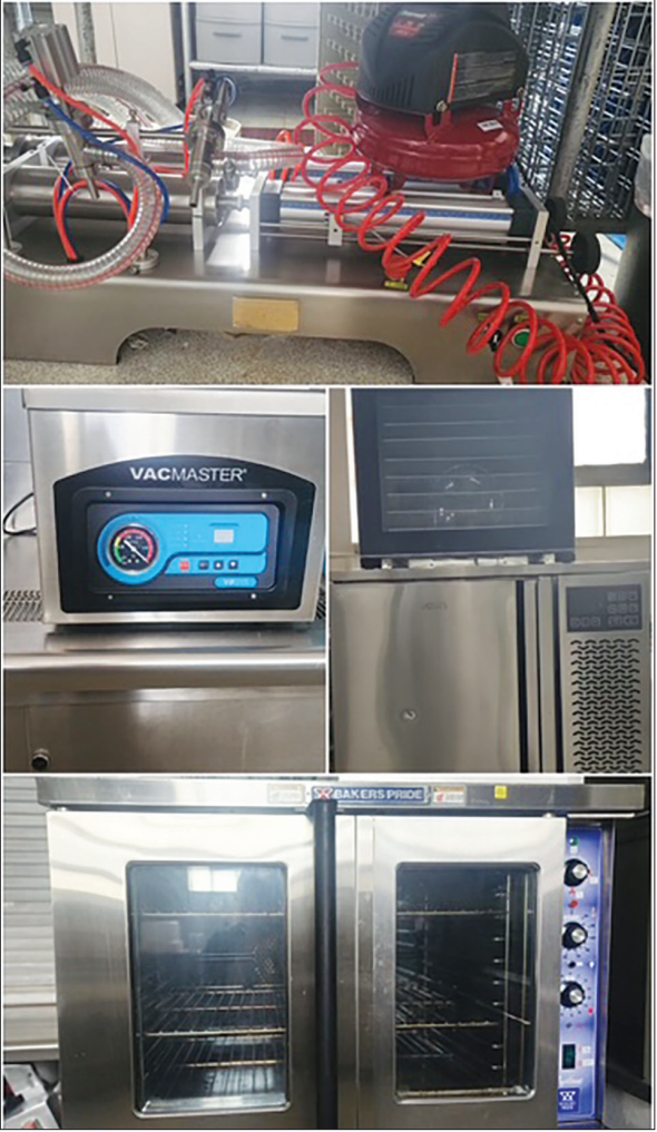
Pictured are the “state of the art” machines installed in the kitchen of the Uptown Event Center. These machines are available for public use.
