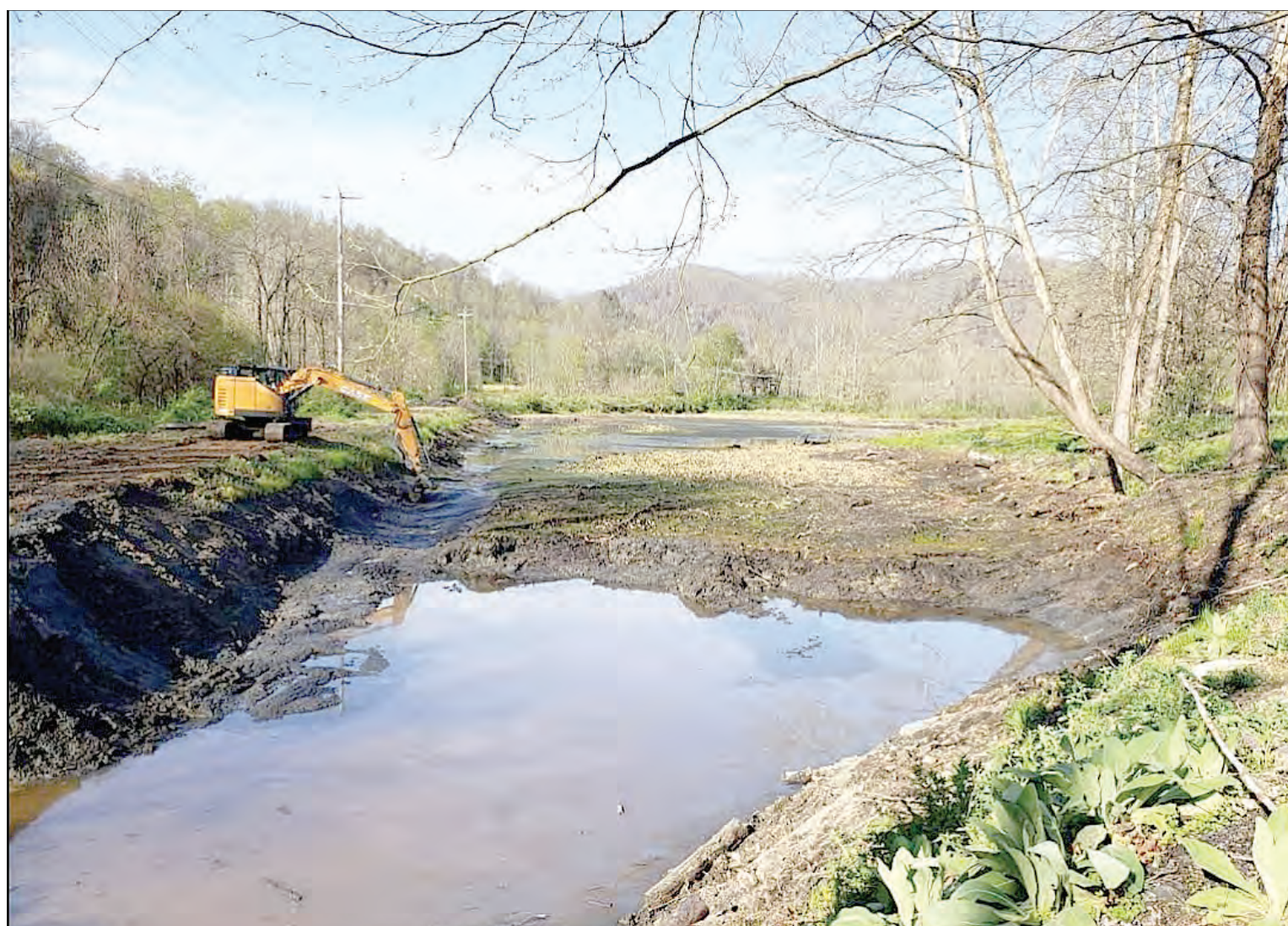
The starting stages of Pulp Mill Pond Restoration Project. Photo courtesy of City of Parsons Facebook page.
