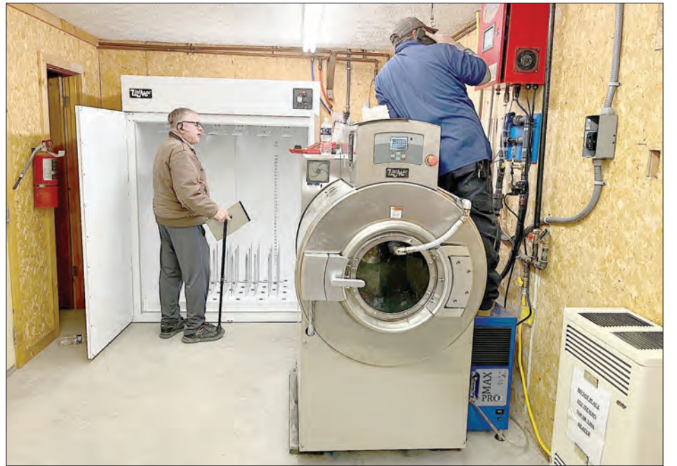
CVVFD Chief Robert Metzger inspected the new drying cabinet designed to get clean gear back in service as quickly as possible. The new, high-tech washer and drying system will make gear safer for first responders by removing harmful substances.
