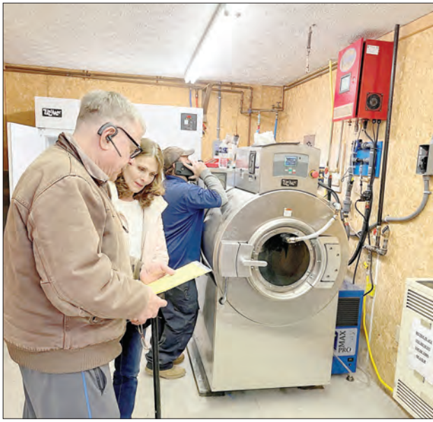
Photos courtesy of CVVFD CVVFD Chief Robert Metzger and Company 30 firefighter Diane Beall checked the specifications of the new units as they were installed last week.
