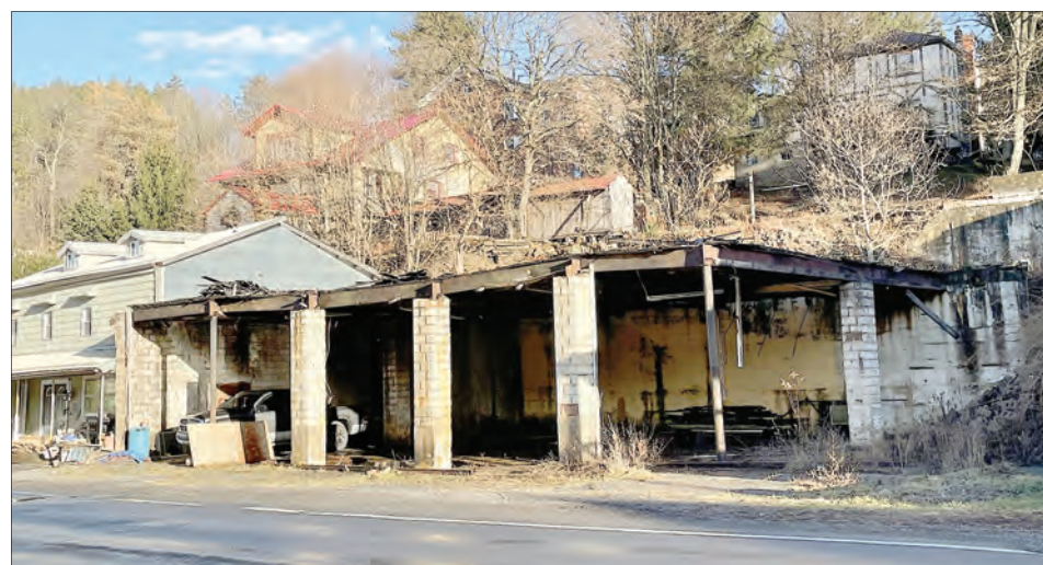
With the passage of an ordinance establishing minimum maintenance standards for buildings, the city of Thomas looks to remove more than a dozen structures, including the century-old Milkint Garage, which collapsed in March 2010.
