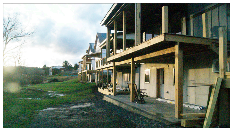
The houses under construction in the Riverwalk project were not included in the filing to condemn by the City of Davis. 12 lots constituting the project's Phase Two and the roadway for the development were included in the City of Davis' filing at the Tucker County Courthouse.
