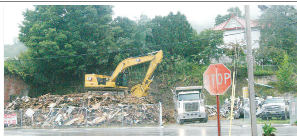
A now vacant lot on Main Street, pictured during demolition in September of 2023, is the site of a housing and commercial project in the City of Parsons that was the subject of debate during a recent City Council meeting.
