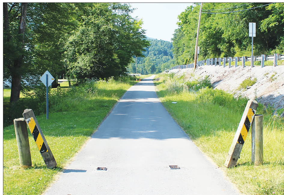
Barriers are being replaced along the Allegheny Highlands Trail in Tucker County. The old wooden barriers are being replaced with new, shorter barriers to assist bicyclists in passing through.
