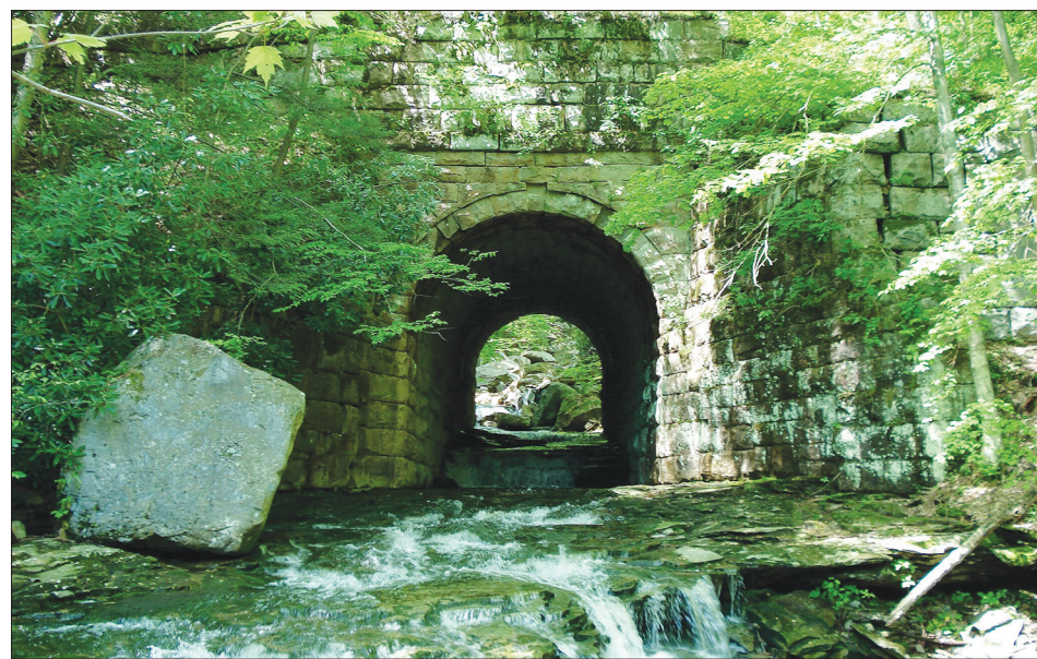
Big Run Culvert before the landslide. Photo from wikipedia courtesy Judy Rodd.
