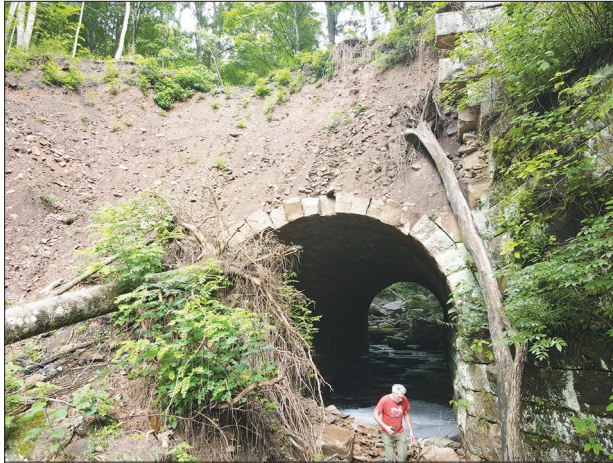
A landslide has damaged the Big Run Culvert along the Blackwater Canyon Trail. Photo courtesy Stephen Strother.
