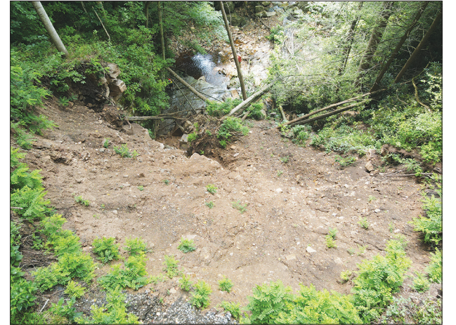
The landslide on the Blackwater Canyon Trail has damaged the keystone on the Big Run Culvert, pictured. Photo courtesy Stephen Strother.
