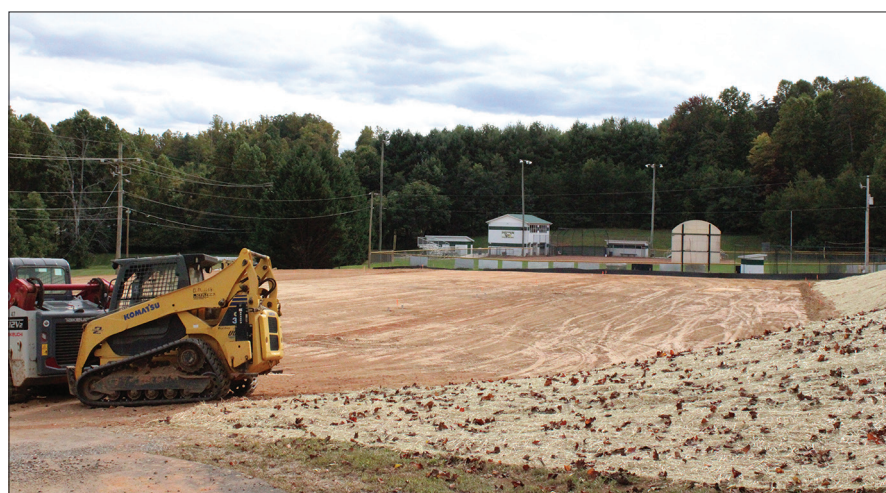
New tennis courts are being built at Patrick County High School. Once completed, the new courts will allow the school to host matches again. (By Pat Delaney)
