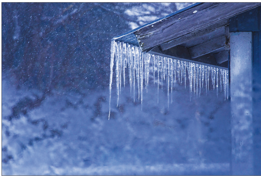
Snow-covered roofs and landscapes can be beautiful, but also dangerous if conditions that cause ice dams to form are not addressed.
