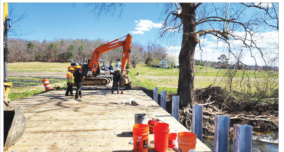
Crews with the Virginia Department of Transportation (VDOT) have been replacing a bridge on The Hollow Road, the Ararat River Bridge, because of flood damage. (By Mary Dellenback Hill)
