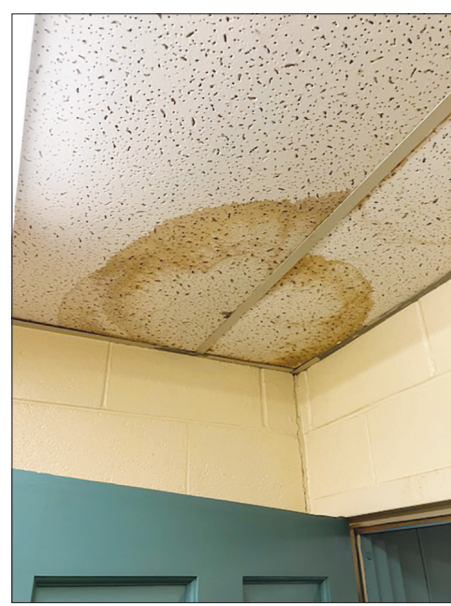
Ceilings on the first floor of Martinsville's Municipal Building sustained damage due to an HVAC leak, prompting the temporary relocation of the General District Court judge and clerk's offices.
