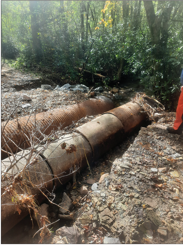
Exposed culverts blocked passage of Panther Creek Road.
