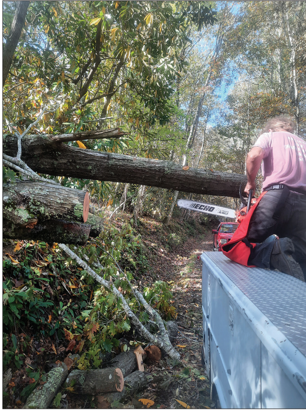
Undeterred, group members prepared to cut trees on portions of Panther Creek Road that were accessible.
