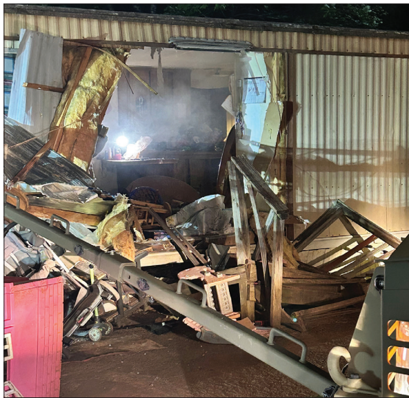
A section of the exterior wall is missing from a home on Norwood Drive following a standoff on July 24, which ended with the arrest of Chase Thomas Fielder.
