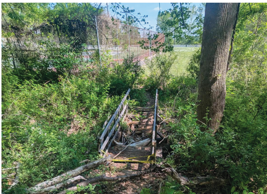
The Woodland Trail bridge at Spencer-Penn Centre is set to be rebuilt, restoring safe, full access to the trail loop.
