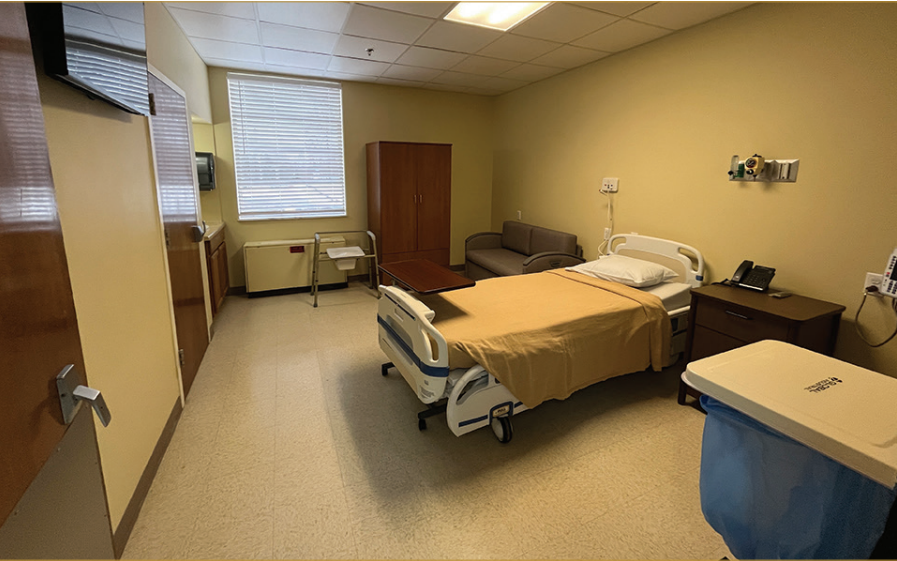
Newly renovated patient rooms include an HVAC register that is controlled by patients.
