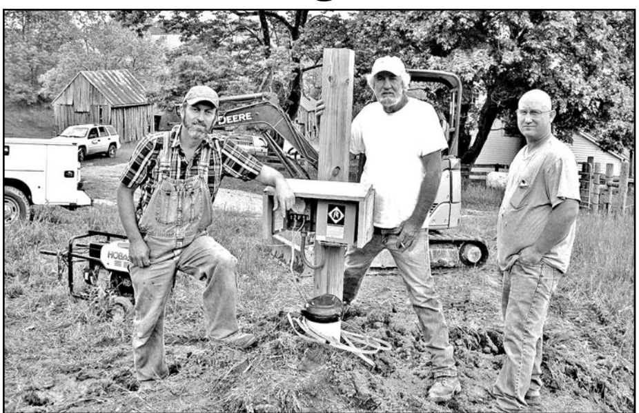
A new well being installed after cattle have been excluded from the stream. SUBMITTED PHOTO
