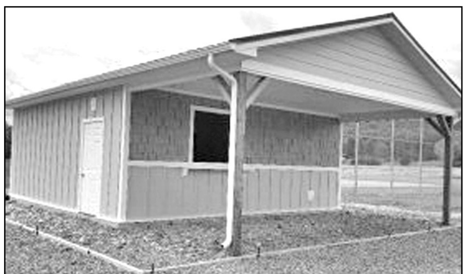
The Field of Dreams continues to build as they just finished their new concession stand.
