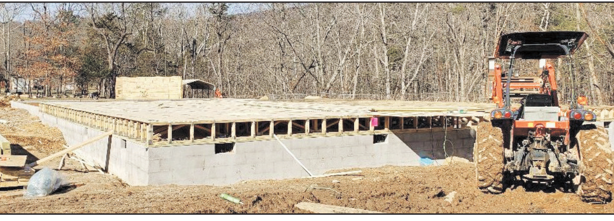
Lighthouse Baptist Church has had a vision to build an addition for a while, and now the dream is becoming reality with the working hands of many people.
