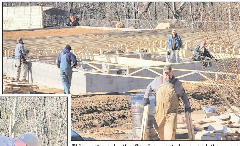
This past week, the flooring went down, and they were pleased to see so much completed.
