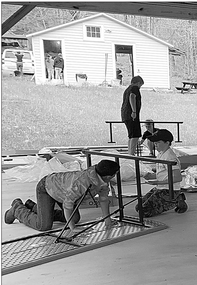
LUKE TAYLOR, COLETON Birley, Levi Hill and Victor Dean construct picnic tables for the new pavilion at Pocahontas County 4-H Camp during clean up day.
