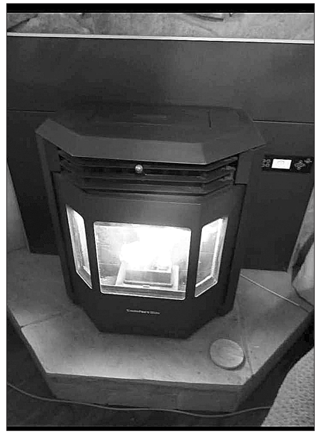
A PELLET STOVE running off of a battery backup, inverter or generator can be a wonderful source of heat during a long winter’s night without power. Photo by Richard Phillips
