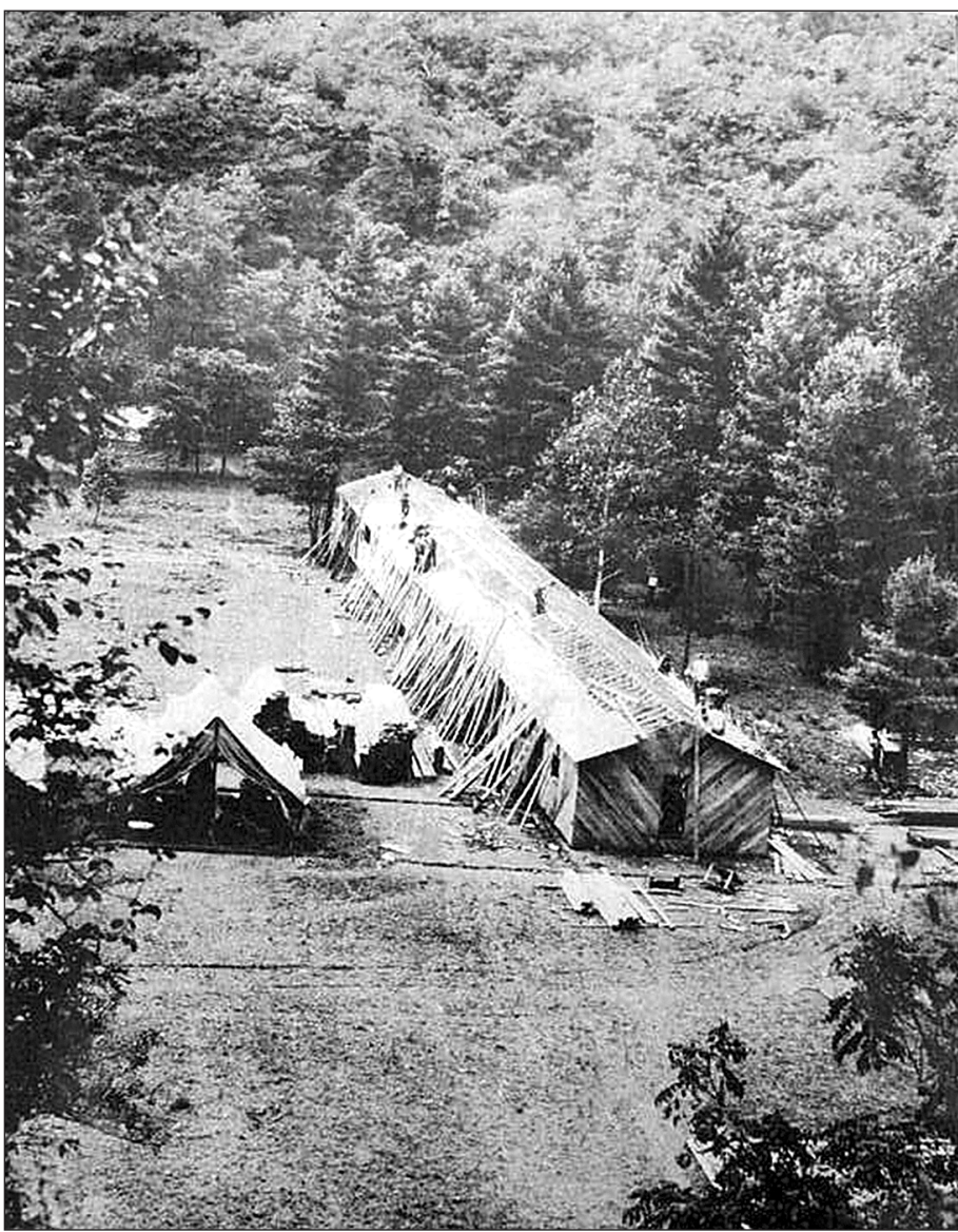
BARRACKS ARE UNDER construction at Camp Copperhead (F 17) located on Bird Run near Frost, W.Va. This Civilian Conservation Corps Camp was established in 1935. The Superintendents were John Gillis and D. J. Parsons. The project was under the supervision of the U. S. Forest Service. Camp Copperhead closed in October 1937. (Preserving Pocahontas Archives; ID: PHP008042)
