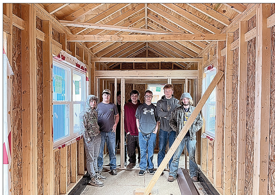
A CLASS OF eight carpentry students at Pocahontas County High School designed and are in the process of building a tiny house. The group did plenty of research to create a living space that is tiny, yet big enough for an individual or small family to call home. Pictured in the house are, from left: Devon Burgess, Devon George, Remington Cook, Joey Cassell, Austin Rider, Caleb Ritter and Justin Lizotte. Not pictured: Jayden Hershman. S. Stewart photo
