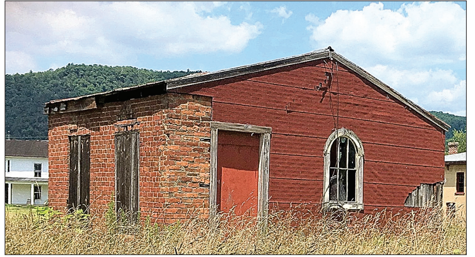
THIS PHOTO, SHARED on Facebook by Denise McNeel in 2022, shows the sad state of the Huntersville Old Clerk's Office before the restoration began. The office was built prior to 1840 when Huntersville served as the first county seat of Pocahontas County.
