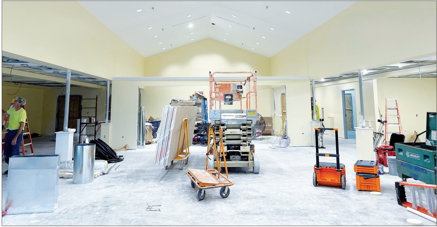
Work continues on completing the day room, designed to provide more light and space for Pendleton Manor residents.
