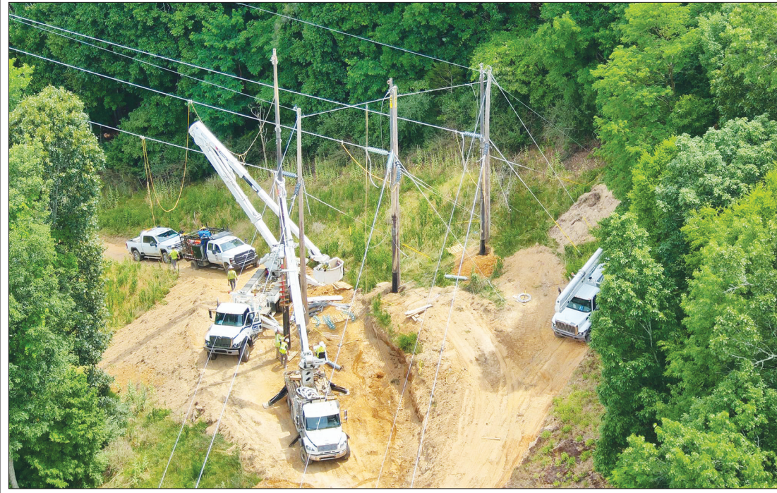
Much of Pendleton County faced a day without power this week as Mon Power conducted line repairs. Photo courtesy of Pendleton County Office of Emergency Management.
