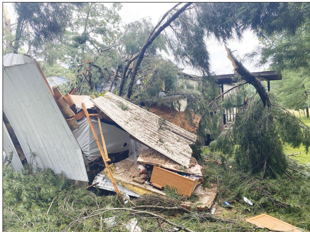
A mobile home/cabin structure off of Sweedlin Valley Road received heavy damage from the winds.
