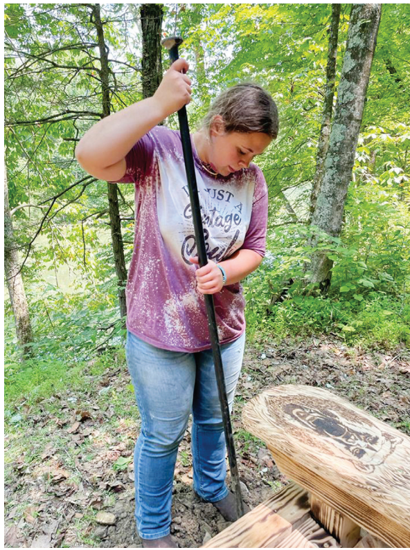
McKenzy uses a spud bar to get the air out of the concrete.
