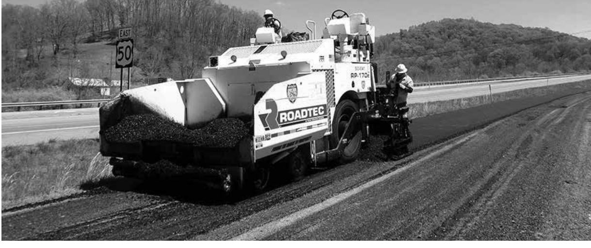
West Virginia Department of Transportation crew members apply new pavement to a stretch of U.S. 50.
