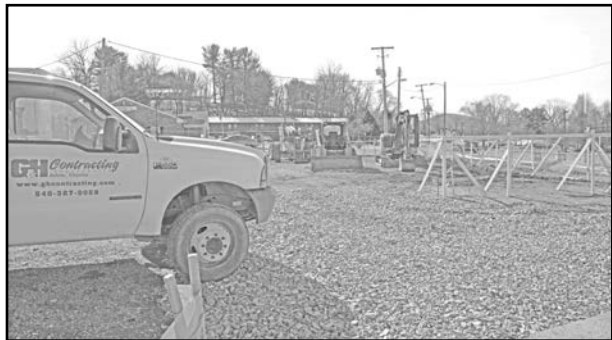
Construction is underway on a new Bank of Botetourt branch on Pollard Street in downtown Vinton.
