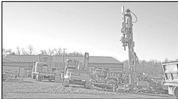
Expansion is underway at the Vinton Rosie's Gaming Emporium, which remains open during construction.
