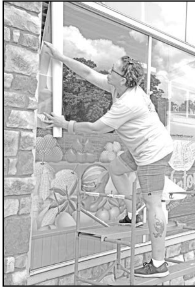
Sun Solutions employee Nancy Rogers installing the window decals at 121 West Lee Avenue in Vinton.
